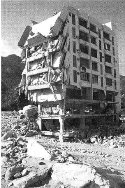
Fig. 2. Debris flow damage to an apartment building in Caraballeda, Vargas, Venezuela, occurred in January 2000. Debris flows passed through the first two stories of this building.
