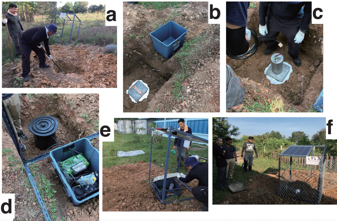
Photo 1. Snapshots of a series of a deployment process. (a) Digging a sensor hole. (b) Making up a basement. (c) Setting up a sensor with determination of the north-direction and leveling. (d) Putting a plastic bucket on the sensor and setting up the data logger, battery, etc., in the plastic box. (e) Fixing a solar panel and closing the logger box cover. (f) Completion of deployment. The station was enclosed with a wire-mesh fence.
