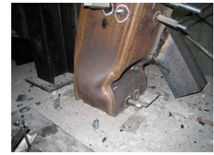
(c) 1階柱脚の局部座屈
